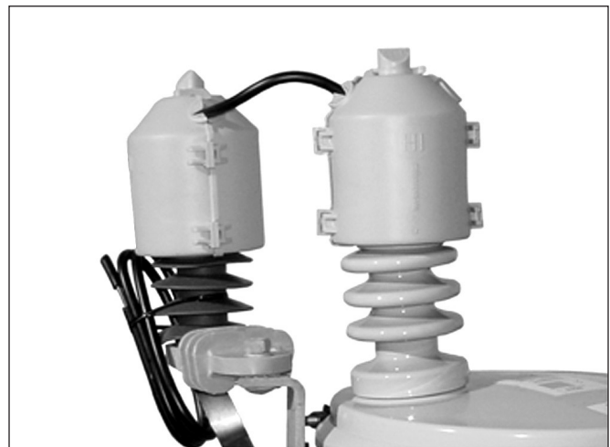
Figure 1: 2140 Wildlife Protectors installed on overhead distribution transformers.
