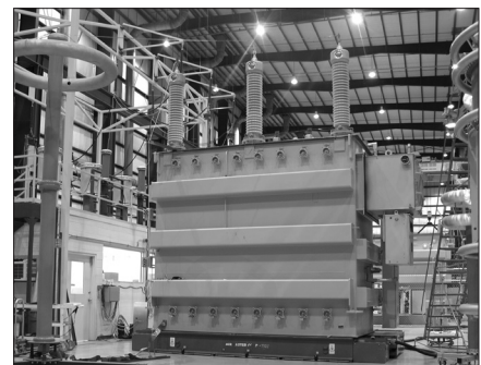
Figure 12: Electrical test station
